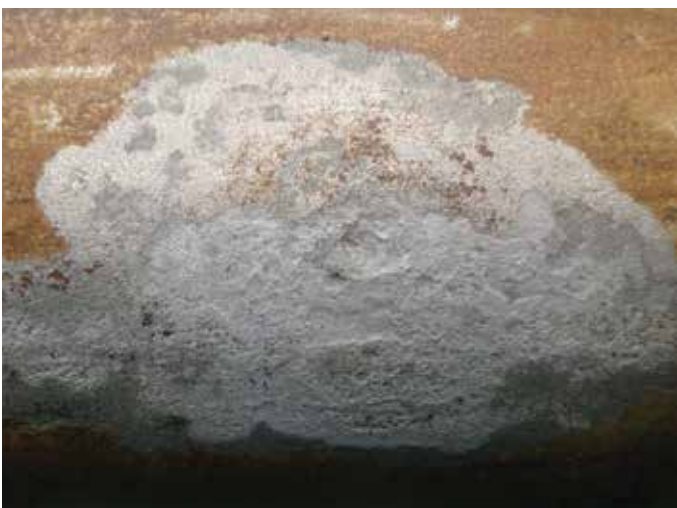
Fig 5. Close up of the deepest area of the localised corrosion (Pipe A)
