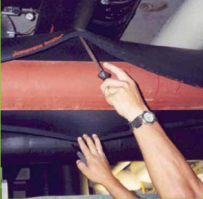
Fig 7: This cold water pipeline has been protected by Armaflex for 20 years - the picture shows maintenance inspection of the original system.
